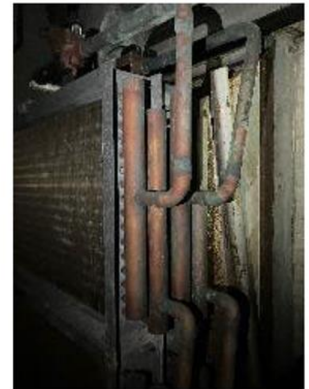
Image 2: Failed Heat-Recovery Coil
